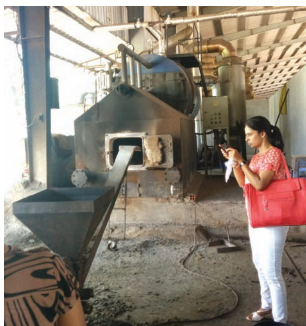
Plate 7.5: Boiler & Steam Generation- Vietnam
