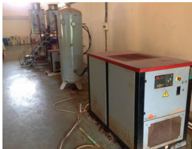
Plate 7.23: Compressor of peeling machine
